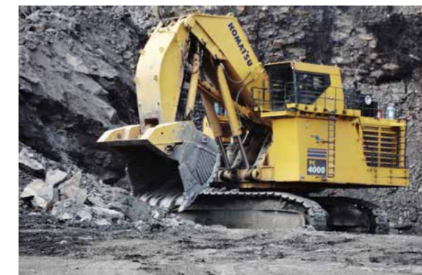
PC4000 hydraulic excavator performing hard rock surface mine operation with Hensley GET system
